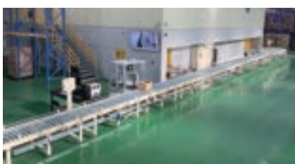
E Plant : E-Beam Irradiation Facility
